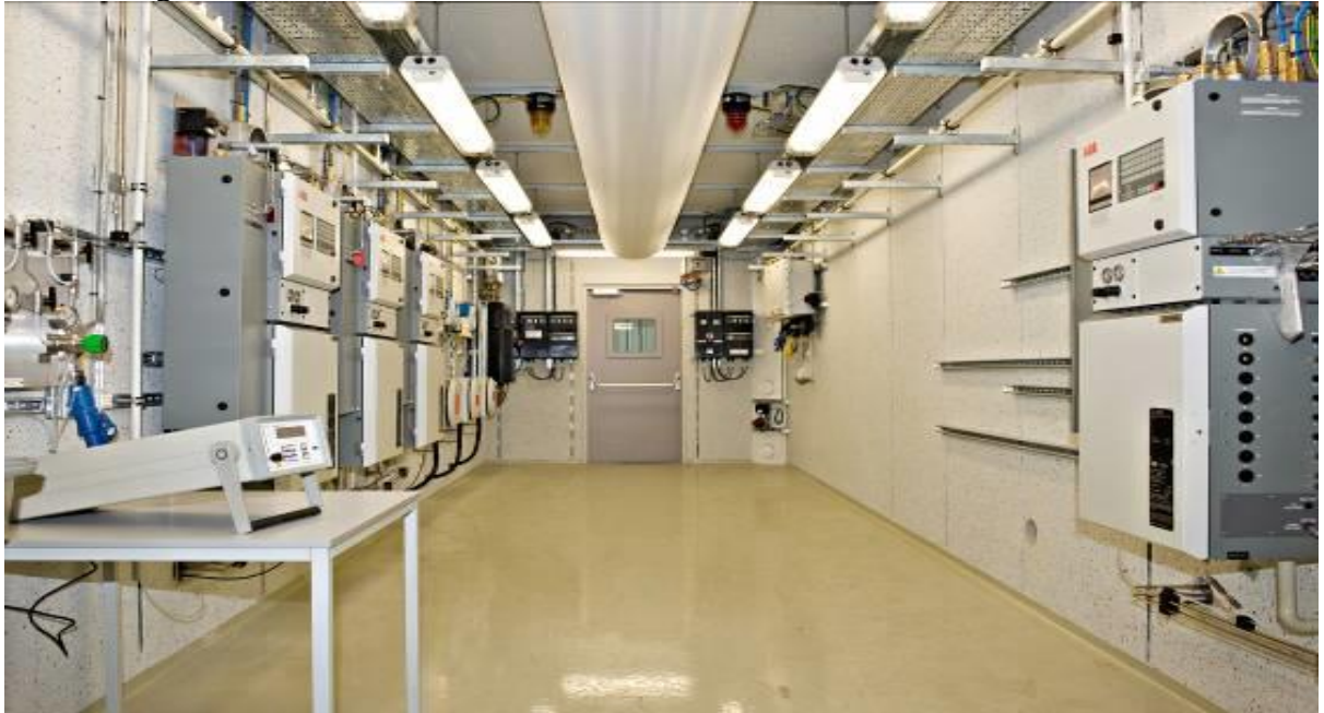
FIGURE 1. TYPICAL ANALYZER HOUSE COURTESY PETROCHEMICAL PLANT
