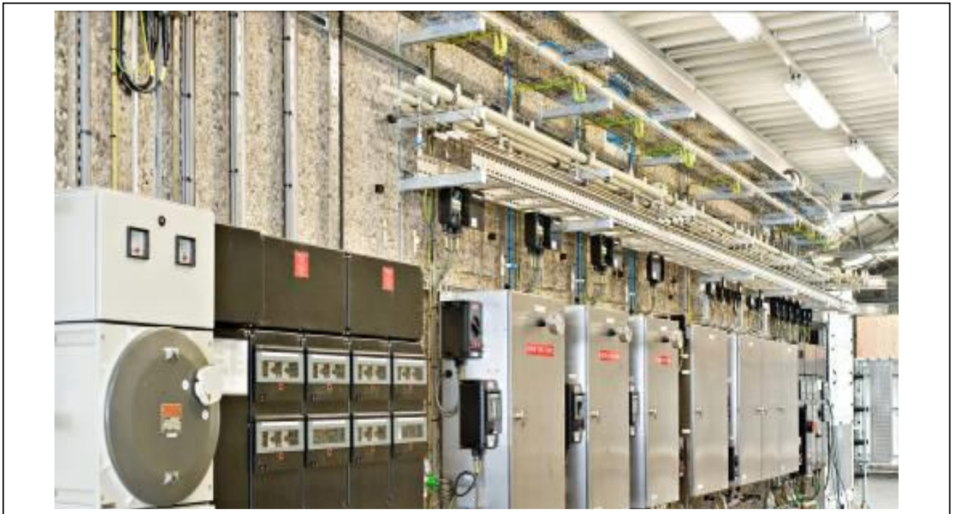
FIGURE 2. TYPICAL SAMPLE CONDITIONING AND SAMPLE HANDLING AREA
